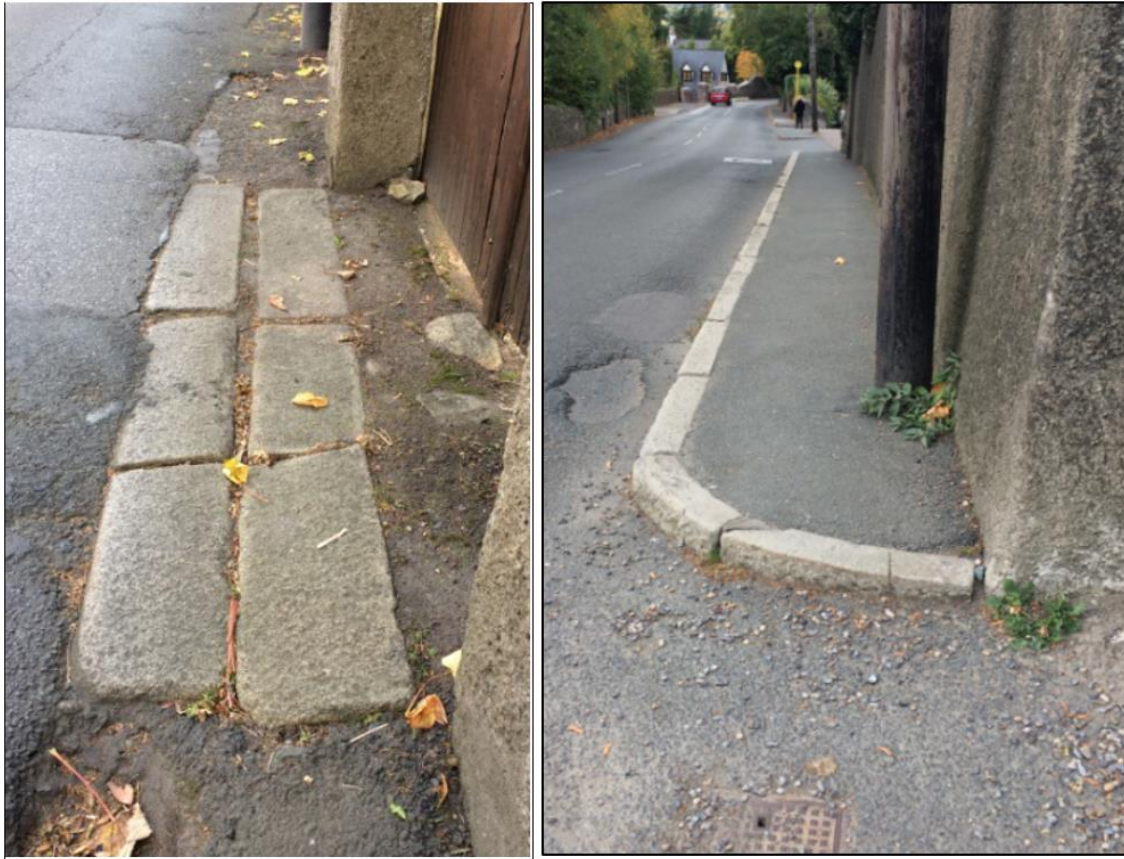
Figure 31 Granite kerbs outside the carriage entrance of the Old Rectory; on the footpath outside Christchurch
