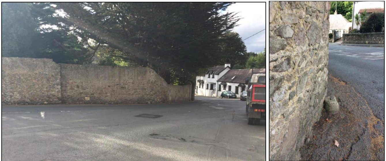
Figure 30 Wall enclosing the Old Rectory; it includes wheel guard stone at the corner
